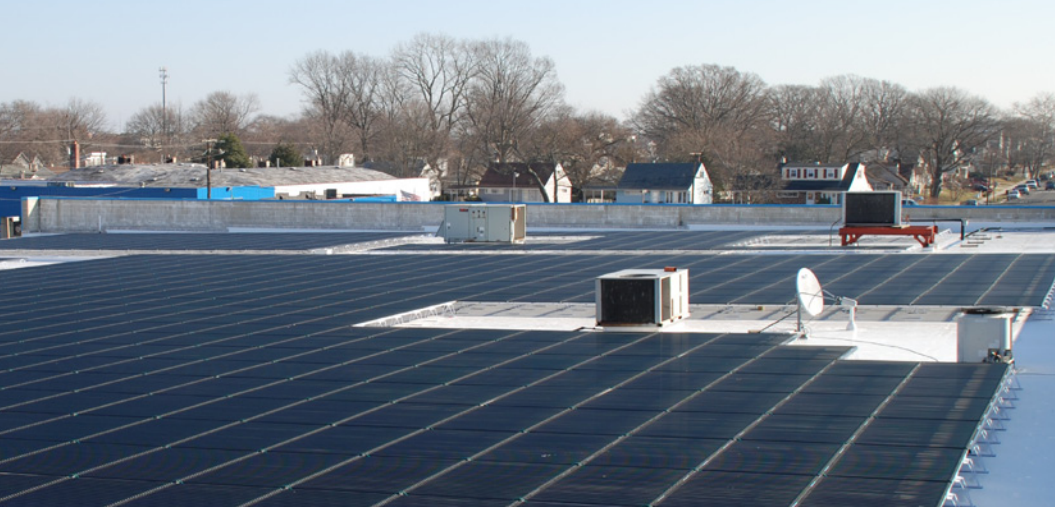
Solyndra panels installed on the rooftop of a Norkus Foodtown store in New Jersey, without the need for anchoring or ballast.
